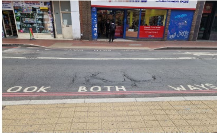
Crossing outside Friars Walk unsuitable for wheelchairs due to road surface defects that have been present for an extended period of time.
